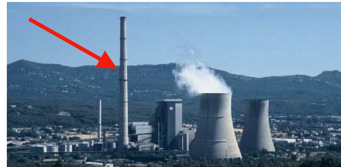
Chimney requiring repairs
