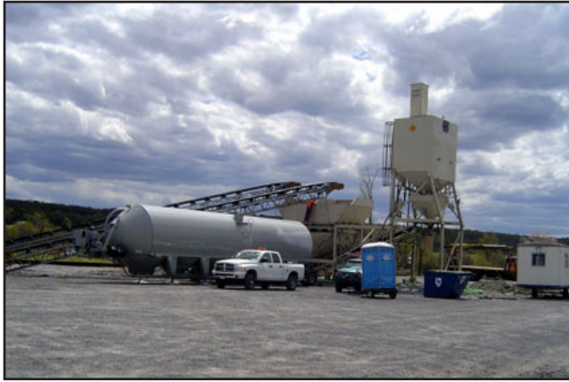
Mobile Concrete Batch Plant
