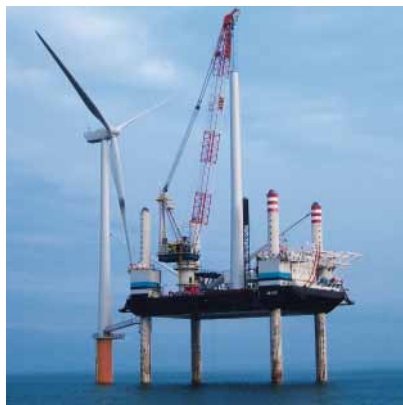
Wind farm // The first turbine is installed at Robin Rigg, an E.ON offshore wind farm.
