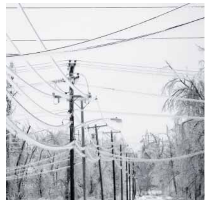
Ice storm // Hurricane Ike and an ice storm cause power outages across Kentucky and many parts of the United States.
