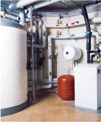
Heat pump with heat storage
