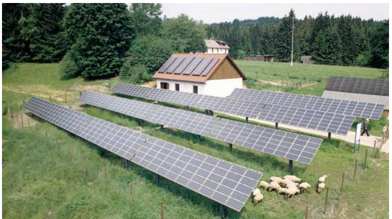
PV installation in rural area of Bavaria
